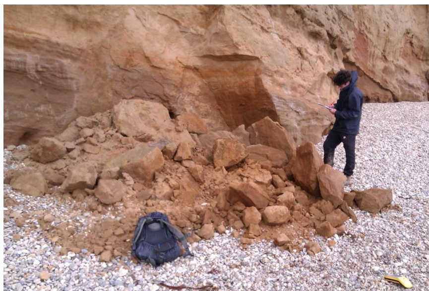
Figure 3.8 Fall type landslide at Red cliff (19). Person for scale and 40L back pack.
