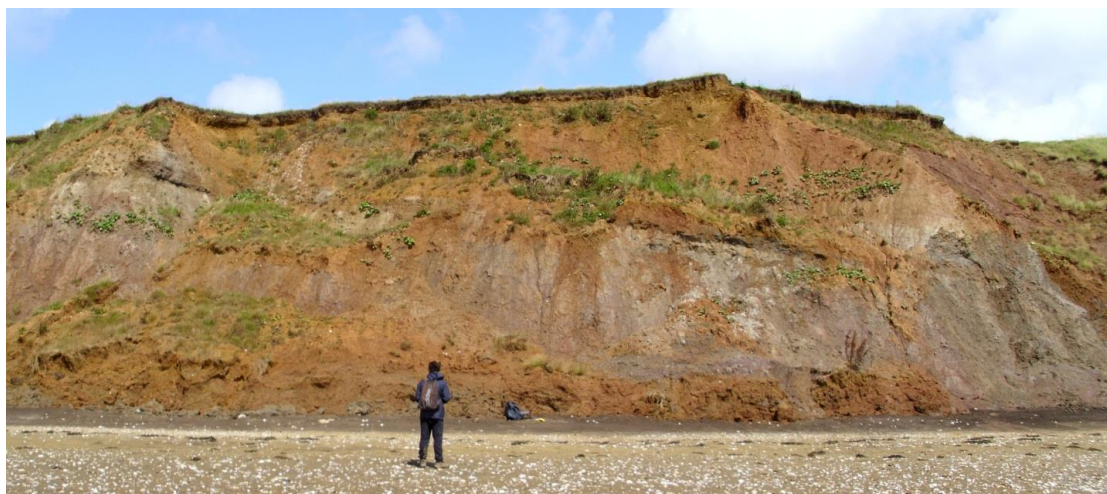
Figure 4.6 Failure occurring in the superficial geology, which is possibly related to increased pore pressures at impermeable layers.
