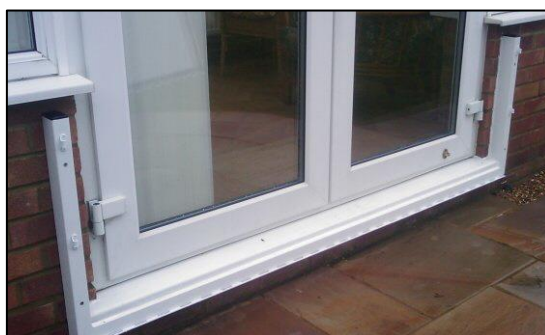
Figure 20: Barrier mount connected to the brickwork below the patio door frame (Flood Wall, n.d.)
