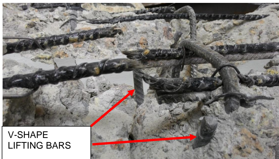
Photo 13: Beam B4 Reinforcement Failure.
