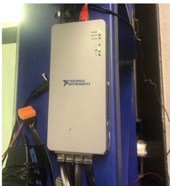
Figure 5: National instruments boxed wired to the strain gauges.
