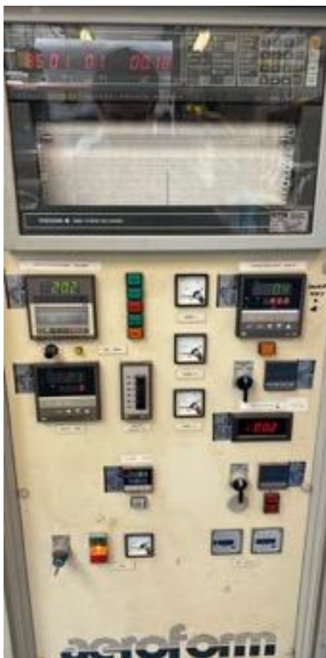
Figure 33: autoclave control panel.
