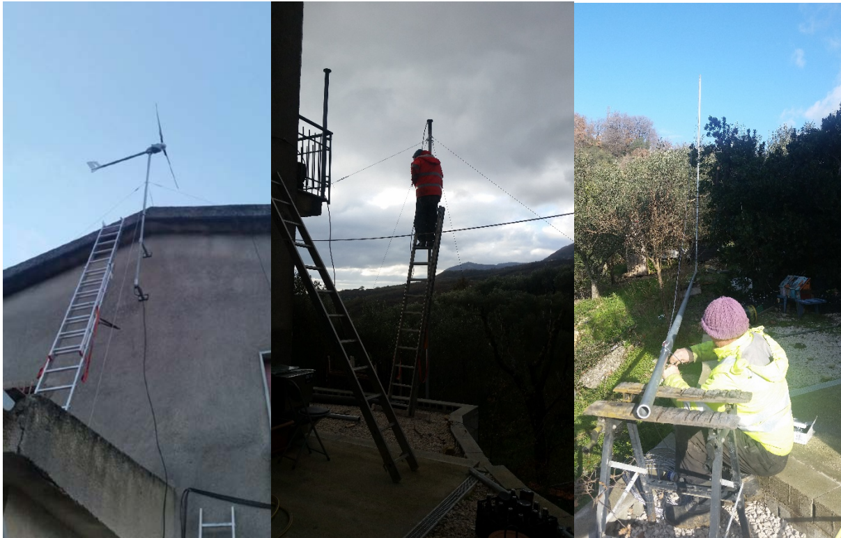
Figure 6.4 Three attempts and arrangements to set up a wind turbine after multiple failures.
